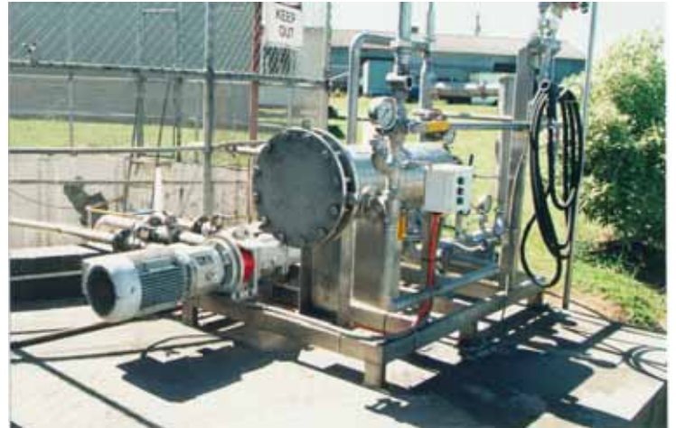
Dairy Effluent Treatment Plant
