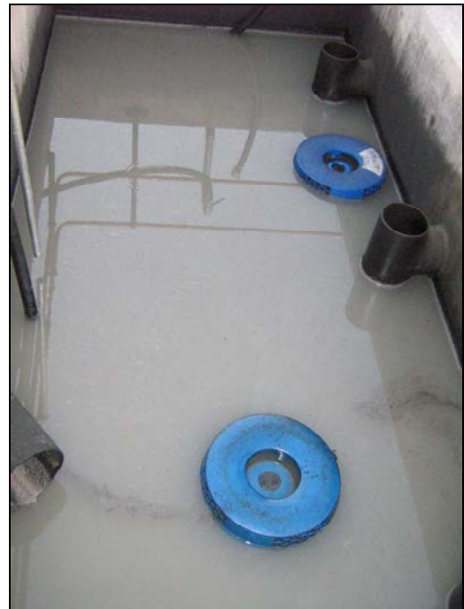
Above: S1 skimmers operating in a pit for a mine site in South Africa
